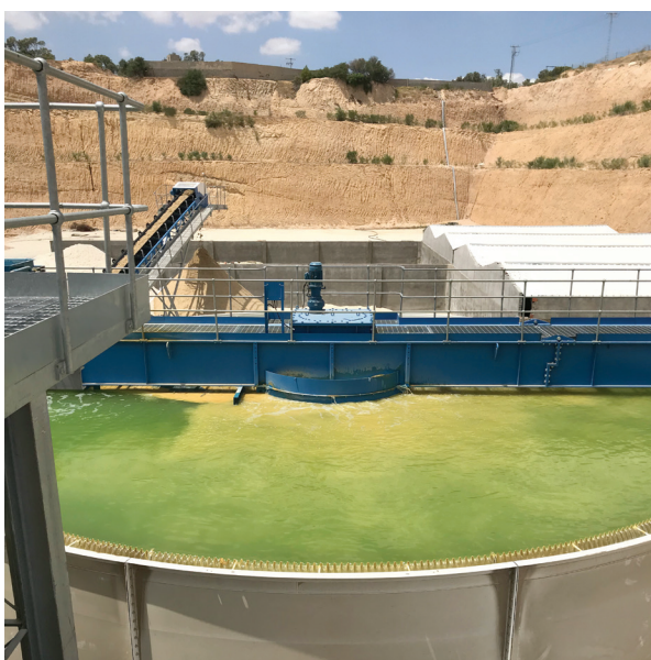
An AquaCycle installation in Tunisia.
