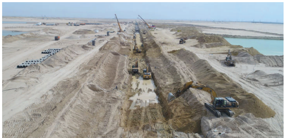
Construction work on infrastructural networks such as roads, rainwater drainage and sanitary services in progress in various sectors of the South Sabah Al-Ahmed City.
